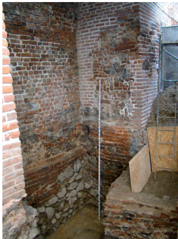
Fig. 8. Gliwice, Basztowa St. Bottom section of the town wall tower, late 15 th –early 16 th century. Photograph R. Zdaniewicz
